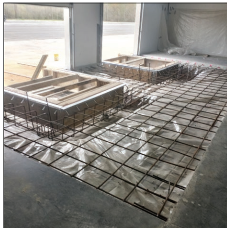
Rebar reinforcement for a set of hydraulic dock leveler pads at a shipping center.
